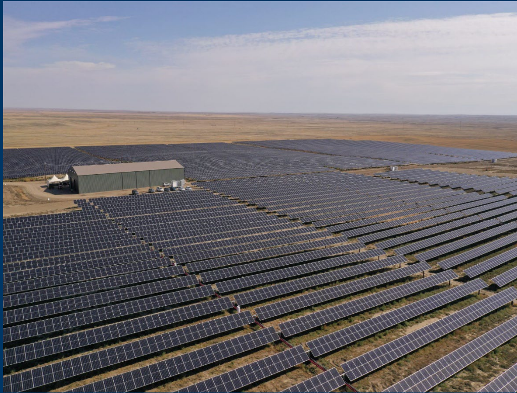
Elemental Energy Chappice Lake Solar Storage
