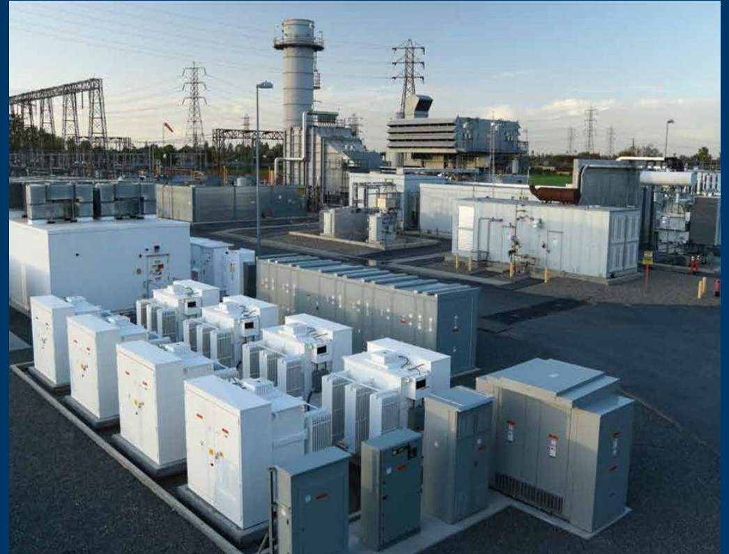
ENMAX Crossfield Energy Center Hybrid Fuel Project
